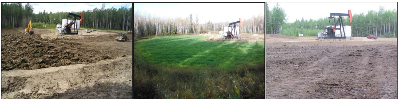
Figure 1. Construction of treatment facility (top), phytoremediation showing grasses in active treatment area (middle), and the decommissioned treatment facility following phytoremediation (bottom).
