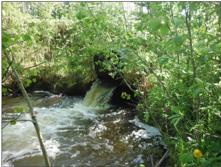
View of the outlet end of the damaged corrugated hanging culvert.
