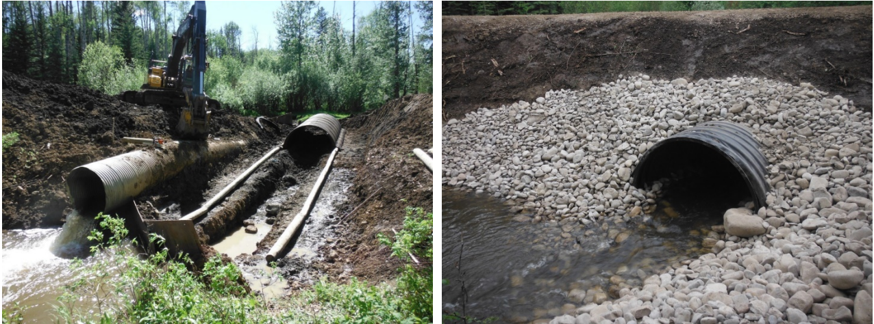
Installation of the replacement system (left), and a view of the outlet end of the newly installed modular culvert (right).
